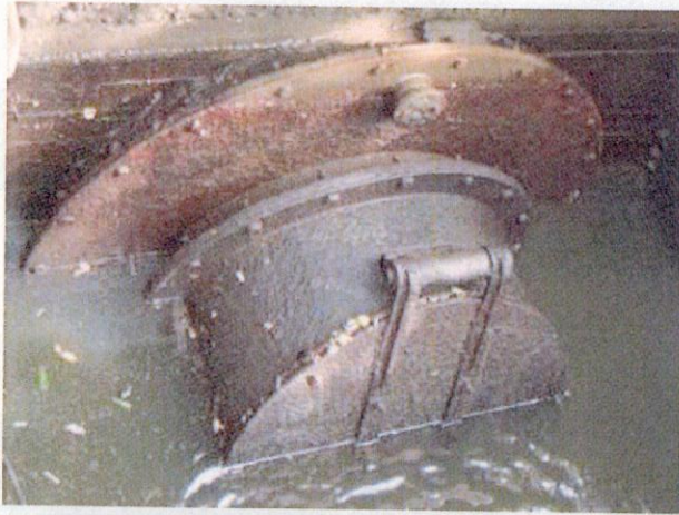
Outfall Flap Valves
