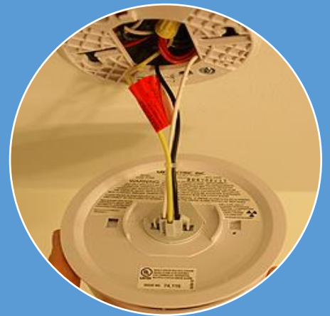
HARD- WIRED CARBON MONOXIDE ALARM
